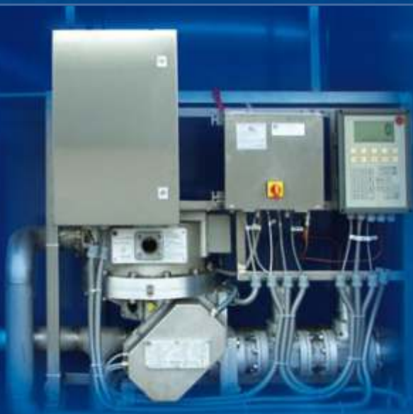
Metering unit TOKA 1200 in a safety cabinet at the public utility company Wuppertal (Germany) installed by the company Schultes GmbH (Düsseldorf, Germany)
