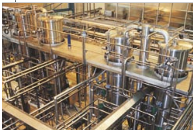
Part of an installation of eight SCC 10,000s
